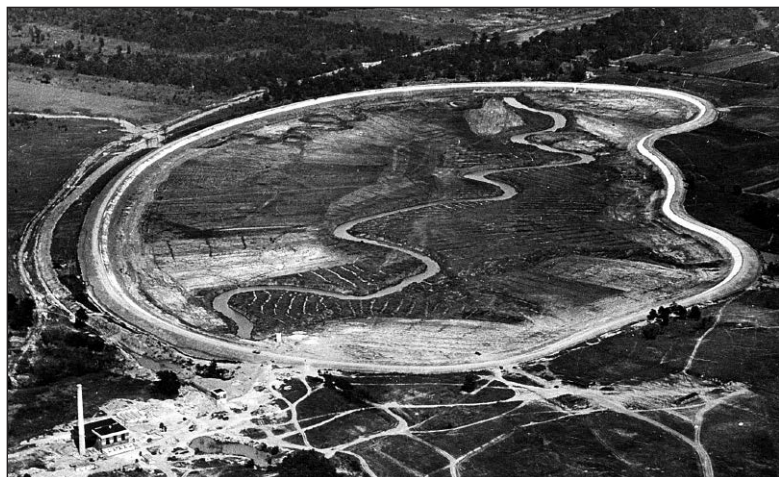
BRING IT ON: The site for the Mohawk reservoir shown here under construction in mid 1923 was chosen because of its above sea level elevation being a mere 75 feet below the top of the soon to be completed Spavinaw dam spillway. Holway persistently proclaimed there was enough drop to provide adequate head for the proposed gravity flow waterline. He did so in the face of stiff opposition from many doubters.
