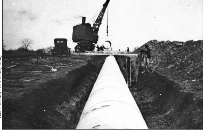
DOWN SHE GOES: It took a 24-ton locomotive crane to carefully lower the ten ton pipe sections into the trench or "cut" as it was called, to join the growing conduit string.
