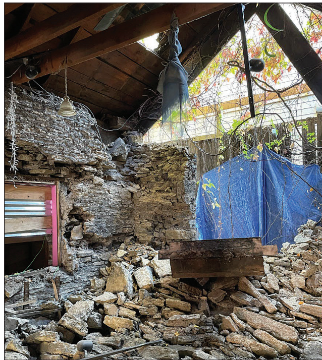
A view of the collapsed wall and damaged roof from the interior of the 170-year-old Justus Ramsey House at 242 W. Seventh St.
