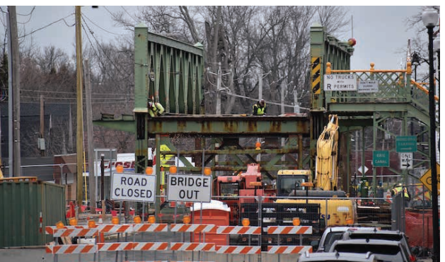
Photo by Tom Rivers: Workers are on top of the deck of the Main Street lift bridge in Albion this afternoon, slowly removing pieces of the bridge.
