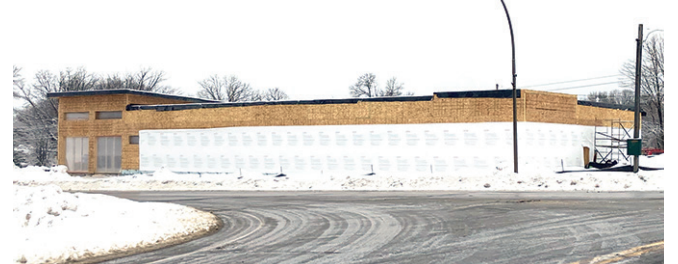
Work continues on the Essentia Health Clinic and Pharmacy building that is scheduled to be completed by spring.
