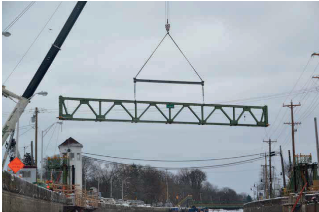
The truss on the west side of the Main Street lift bridge is hoisted on the afternoon of Jan. 27 at about 2:30.
