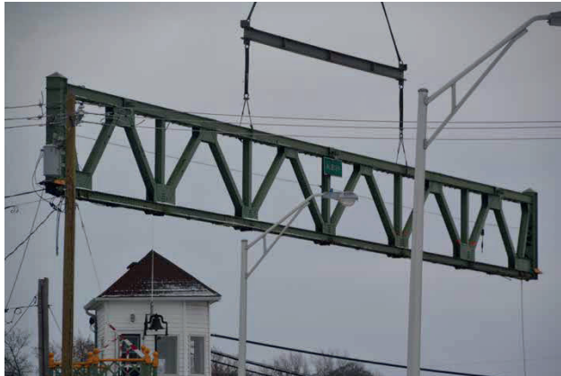
The first one was removed with a crane at about 11:45 a.m. This photo shows the truss over the lift bridge tower.
