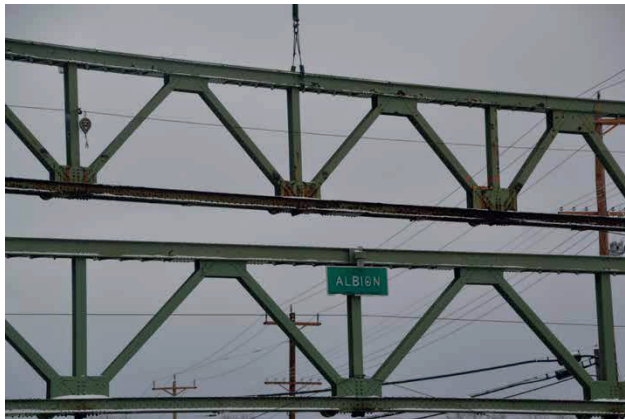
The first truss is lifted at 11:45 on Jan. 27. Many onlookers showed up to take photos and observe a historic day in Albion.
