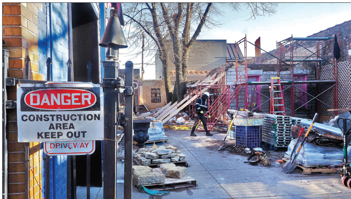
A worker sweeps up on February 16 as the Justus Ramsey House is dismantled on the Burger Moe's patio. PHOTO BY BRAD STAUFFER
