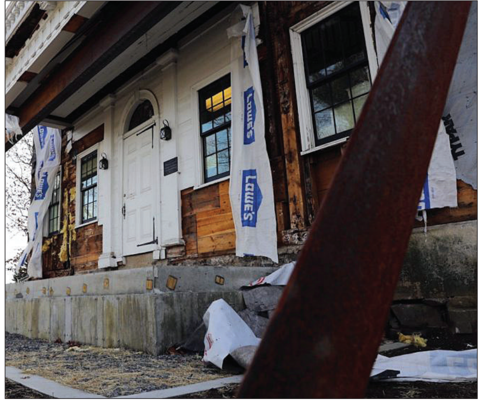
A steel frame holds up the balcony after the support columns were removed for repairs.
