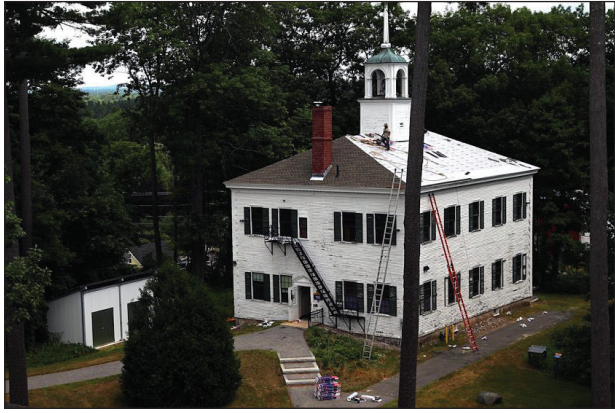
A roofer takes a break from laying new shingles on the Academy Building to check his equipment.
