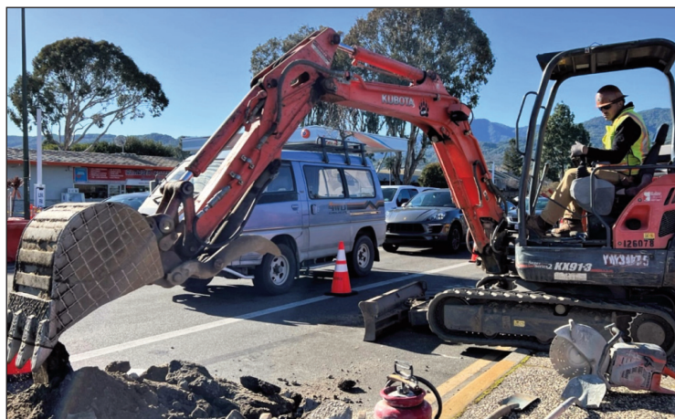
A construction worker uses a backhoe to excavate the roadway on Camden Avenue in January. Photo courtesy of Santa Clara County.
