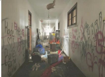
A corridor at College Avenue Elementary riddled with graffiti and trash.
