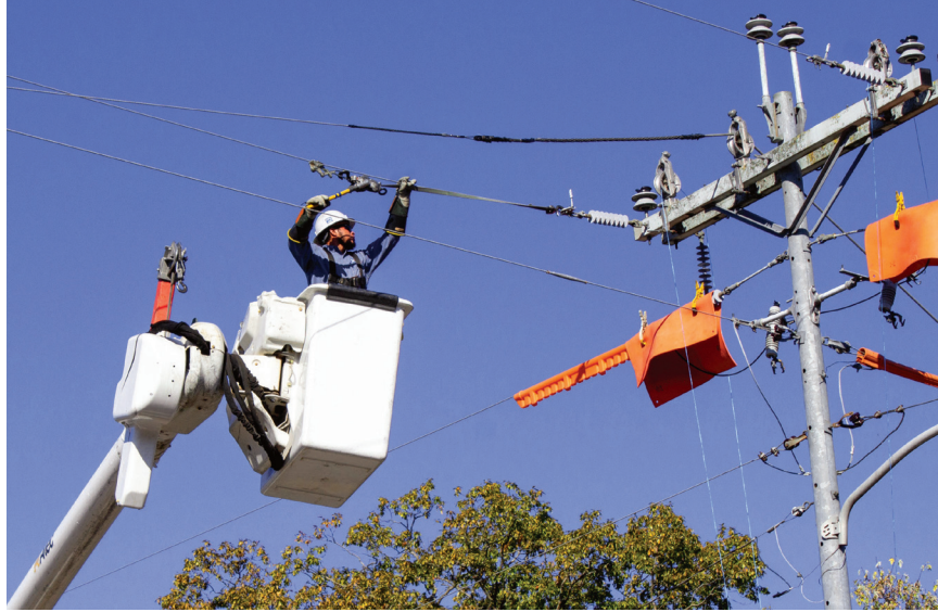
As an apprentice lineman for FPU, Derian Morales performs maintenance on electrical lines.
