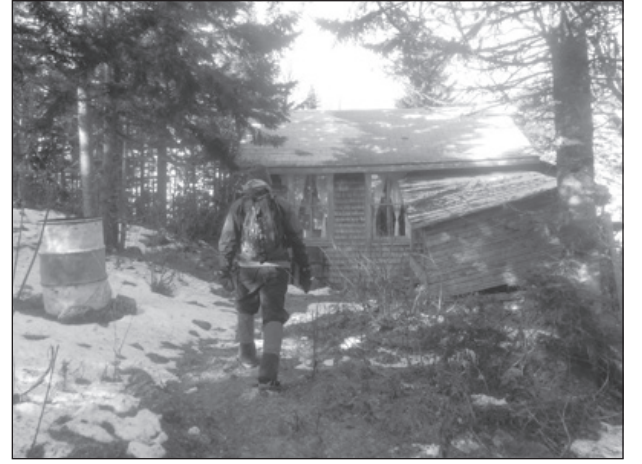
A dilapidated Fire Warden's cabin is located a short distance below the summit
