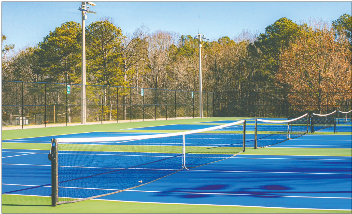
A Northwest Alabama Resource Conservation & Development Council grant allowed for six new tennis courts to be constructed at Killen Park. Three courts have been lined for pickleball. [DAN BUSEY/TIMESDAILY FILE]
