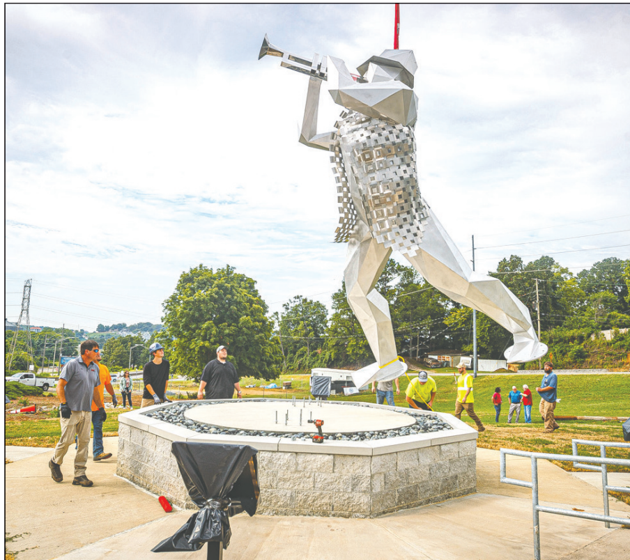
Workers use rope to position the Singing River sculpture as it is installed July 8 at the corner of North Court and Bluff Streets. [DAN BUSEY/TIMESDAILY FILE]
