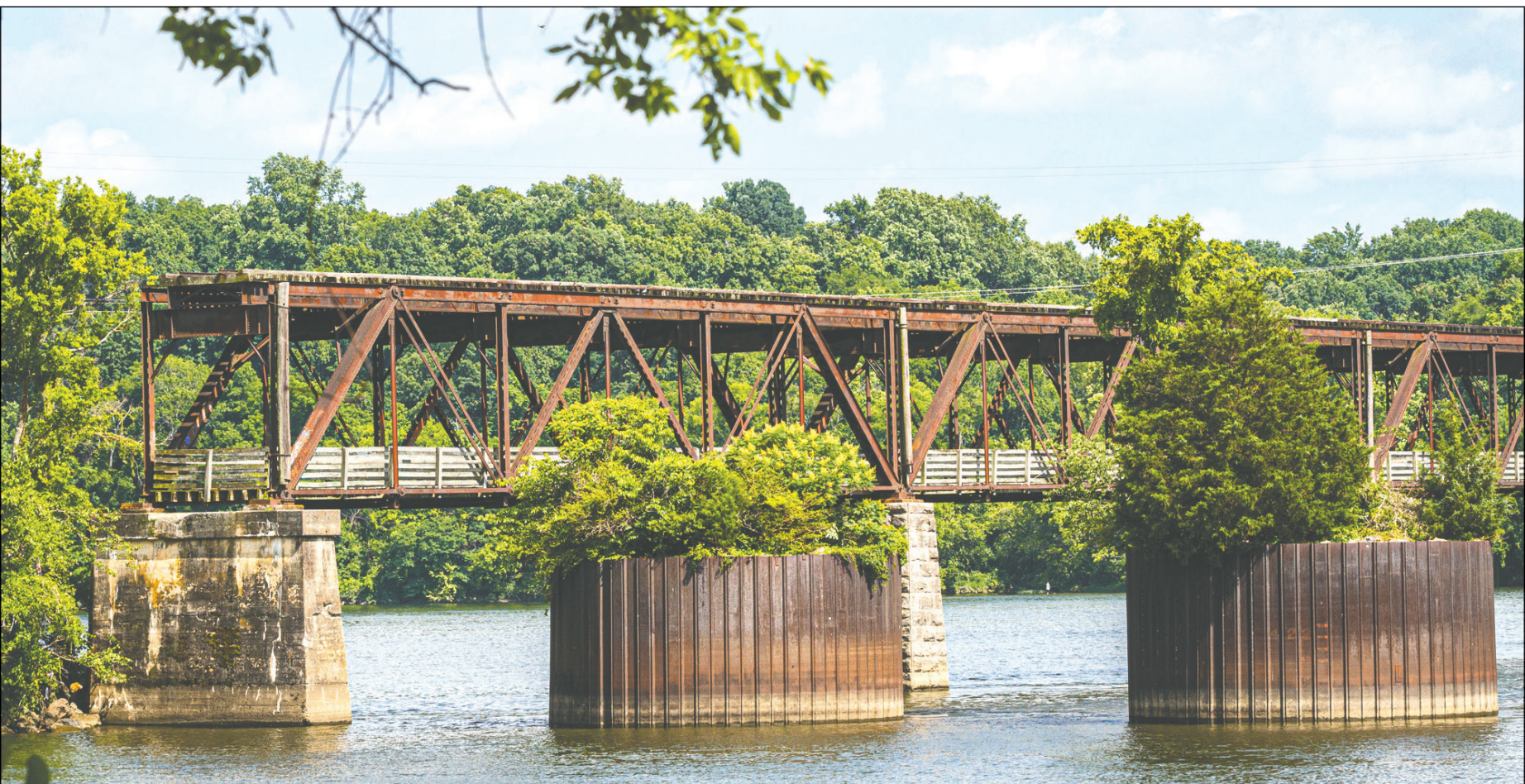
The old railroad bridge in Sheffield has been recently added to the National Register of Historic Places. [PHOTOS BY DAN BUSEY/TIMESDAILY]
