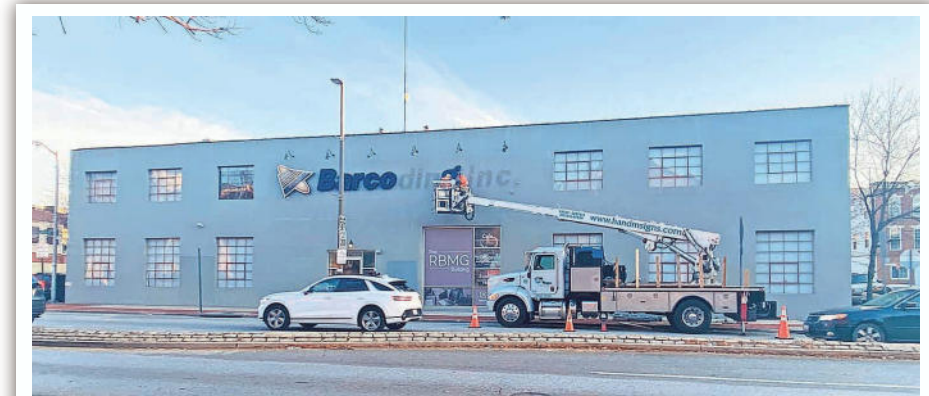
Signage of the prior owner, Barcoding, Inc. is removed from the facade of the building located at 2220 Boston Street in Baltimore in 2023. The RBMG Building was purchased by Dr. Vonnya Pettigrew.
