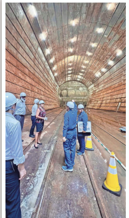
Maryland Delegation visits underground SC Maglev station construction site in Kanagawa Japan to see firsthand how community impacts are avoided and minimized.
