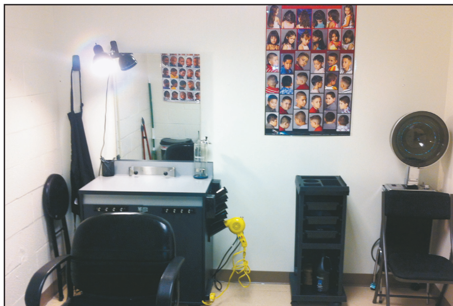
The project at the Phoenix Academy marks R.B.C.F.'s sixth fully installed barber/beauty salon. Photo Credit: Jordan Ulmer
