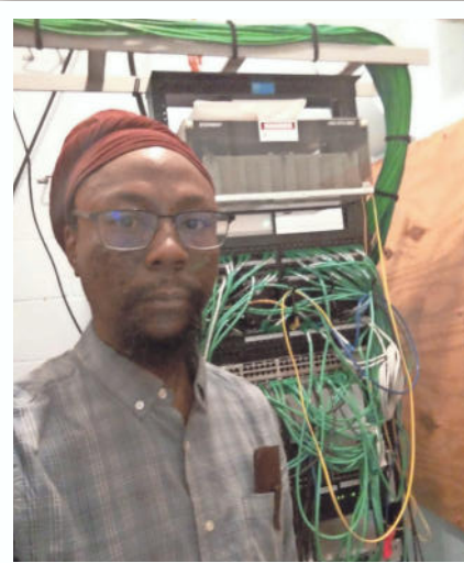
Terrell Freeman-EL in a server room of a client, post installation and testing of multiple network devices.
