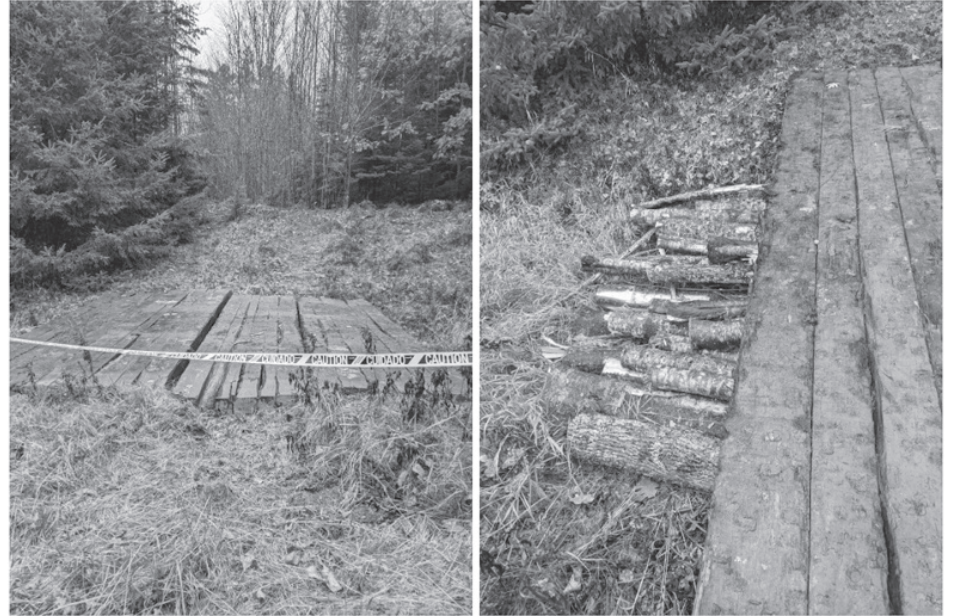
Crossing constructed to access drilling location. Photo credit: Jill Howell, Upstream Watch
