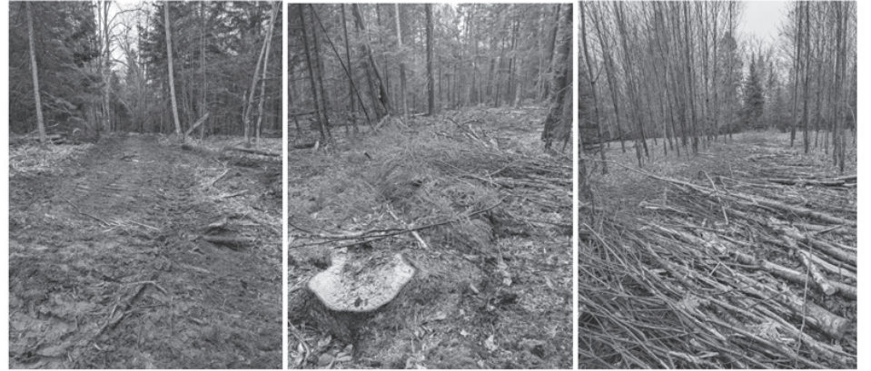
Tree clearing and access path construction. Photo credit: Jill Howell, Upstream Watch
