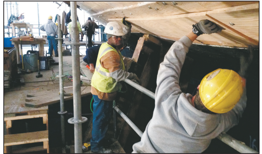
A crew of skilled men and women work long days to restore USS Constellation's wooden hull. When the historic USS Constellation returns to the Inner Harbor on or around February 20, 2015, she will be open daily for public tours as a living classroom and as the flagship of the Historic Ships in Baltimore fleet.
