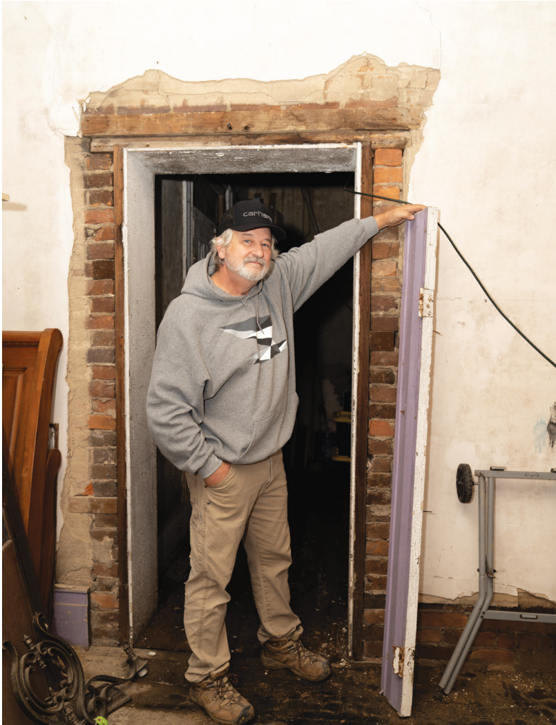
▲ Keith holds a piece of door trim from the living room of their home. This trim is original to the home and was held with square nails.
