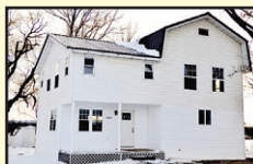
Chittenango $105,000 Remodel in progress. Finished this home the way you want. Chittenango Schools. Peter Denney 247-1910 (D)
