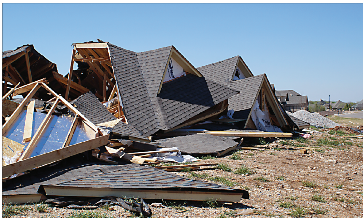
TORNADO AFTERMATH: A photo of one of the two homes in Stone Canyon that was leveled by the March 30 tornado. Both homes were under construction. After the tornado, the community received supplies and volunteer support from neighbors and local organizations, including Owasso Land Trust, Home Builders Association of Greater Tulsa and American Red Cross.
