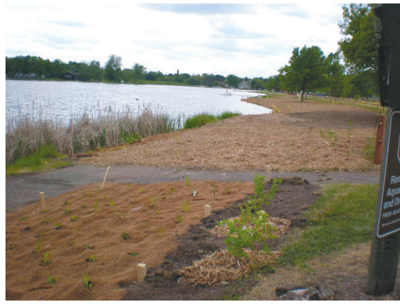
In the summer of 2009, the City of Crosby with Crow Wing SWCD, the Serpent Lake Association, MN DNR and several Master Gardeners installed two rain gardens and a shoreline buffer (pictured above.) A $400,000 project for rain gardens along the westside of the ballfield and the northeast corner parking lot next to the ballfield is now being proposed in Crosby.
