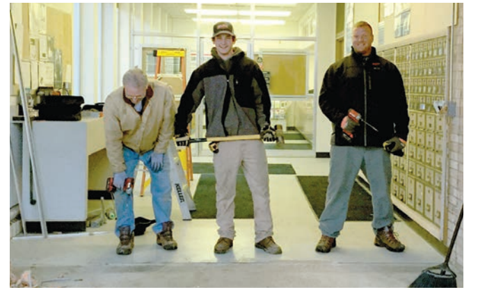
Before the really cold weather hit, the north wall of the Aitkin Post Office, made entirely of glass, was replaced. One morning when customers came to their post office boxes, they found the lobby open to the elements. Working to replace the glass, from Gull Lake Glass, was Bob from Baxter, Cooper from East Gull Lake and Kevin from Lakeshore. Ann Schwartz photo
