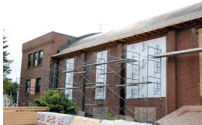
The Aitkin Army is undergoing extensive remodeling to convert it to assisted living units for the elderly.
