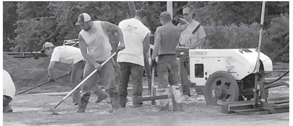
A cement slab was poured recently as construction continues for Aitkin's new Family Dollar Store. The building is going up on Aitkin's main street, Minnesota Avenue South. Ann Schwartz photo
