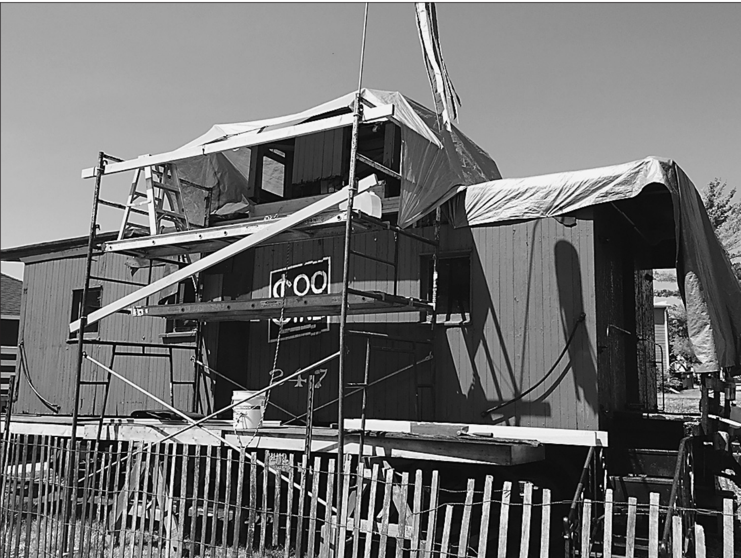
This photo and others adjacent to the Village Report show the progress of the caboose renovation project. Delays in the project will postpone the rededication of the historic railroad car.
