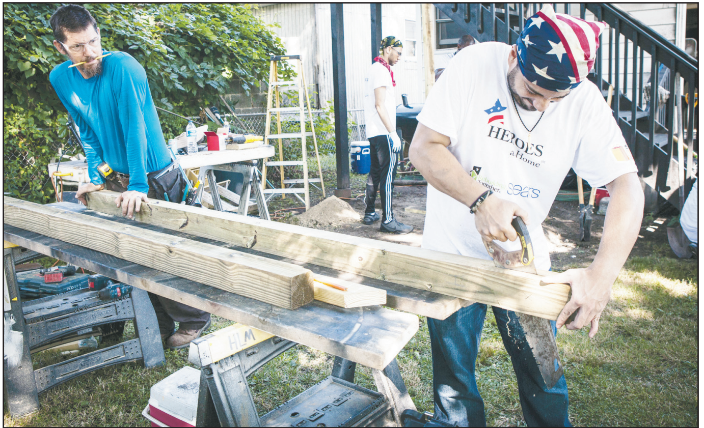
Sears Heroes at Home teamed with nonprofit Rebuilding Together Baltimore as a team of more than 20 Sears volunteers helped repair and renovate U.S. Army and Reserves veteran Charles Faison’s home of 52 years. In addition to the stairs, repairs included fixing damaged ceilings, roof patching, a new Kenmore stove, accessibility upgrades and more.
