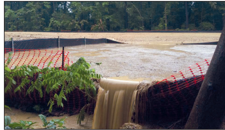
Sediment-laden storm water spilled over the silt fence on July 16. Courtesy photo.
