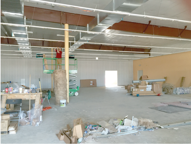
Construction on the new Family Dollar Store in downtown Aitkin is continuing. Last week, electricians installed lights in the interior. Ann Schwartz photos
