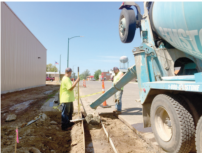
Curb and gutter are poured at the Family Dollar block in Aitkin. Later, signs were installed on the exterior.
