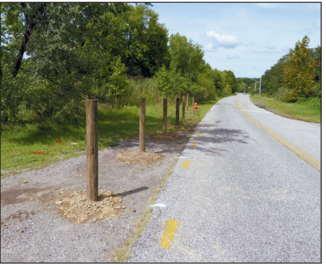
DPW workers began installing the bollard-and-cable fencing on Sept. 1 and are expected to finish by Sept. 15.
