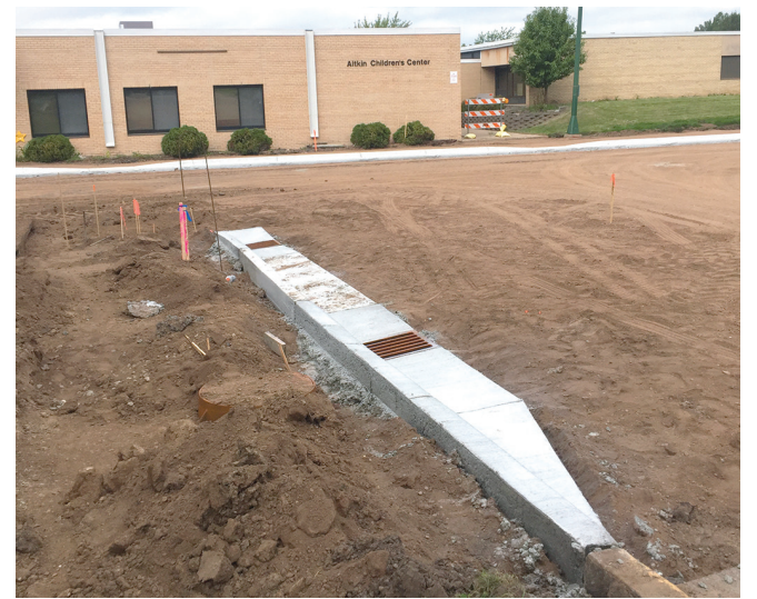
One layer of bituminous and new sidewalks are laid in the area of Rippleside Elementary in Aitkin as a large sewer project nears completion. Ann Schwartz photo
