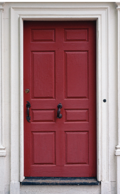
Air leaks around doorways can waste energy and cost homeowners substantial amounts of money.
