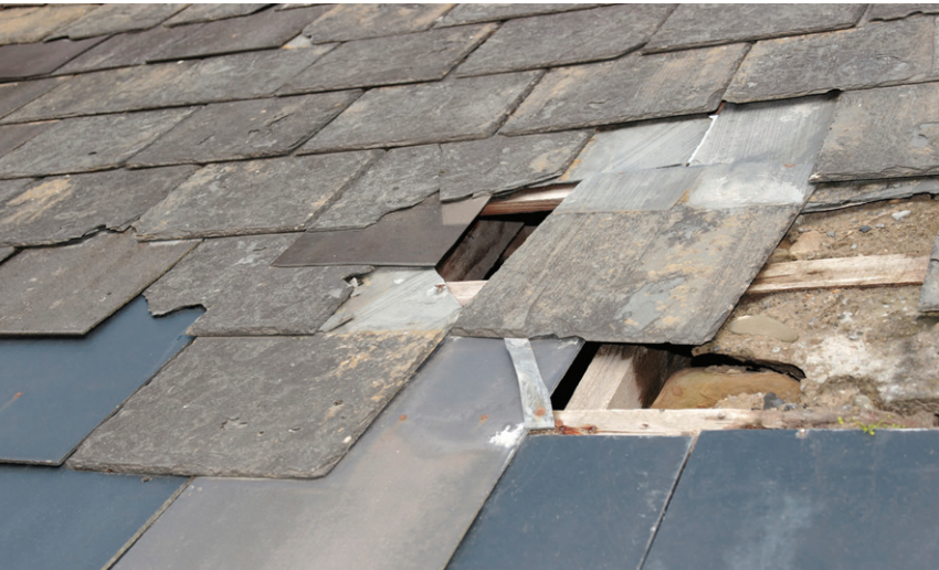
Inspect a roof each fall to get an idea of the potential damage and any necessary repairs that may be needed before nasty weather sets in.
