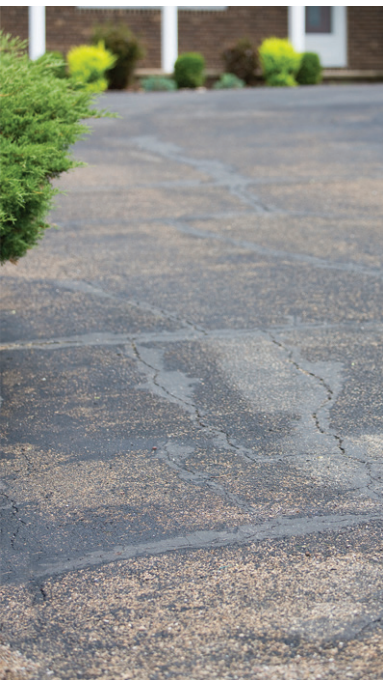
Surface cracks in a driveway may indicate a problem that requires immediate attention.
