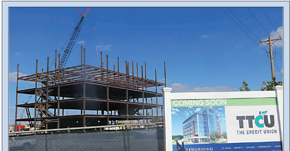
GOING UP: The new corporate headquarters for TTCU The Credit Union is well underway at 9815 E. 81st St. in Tulsa, next to the TTCU Southeast branch. Expected completion is late 2016 for the six-story, 90,000-square-foot facility. Ground was broken on June 25, and officials say that the new headquarters will enable the TTCU team to provide even greater levels of service to the existing membership and to expand membership in years to come.
