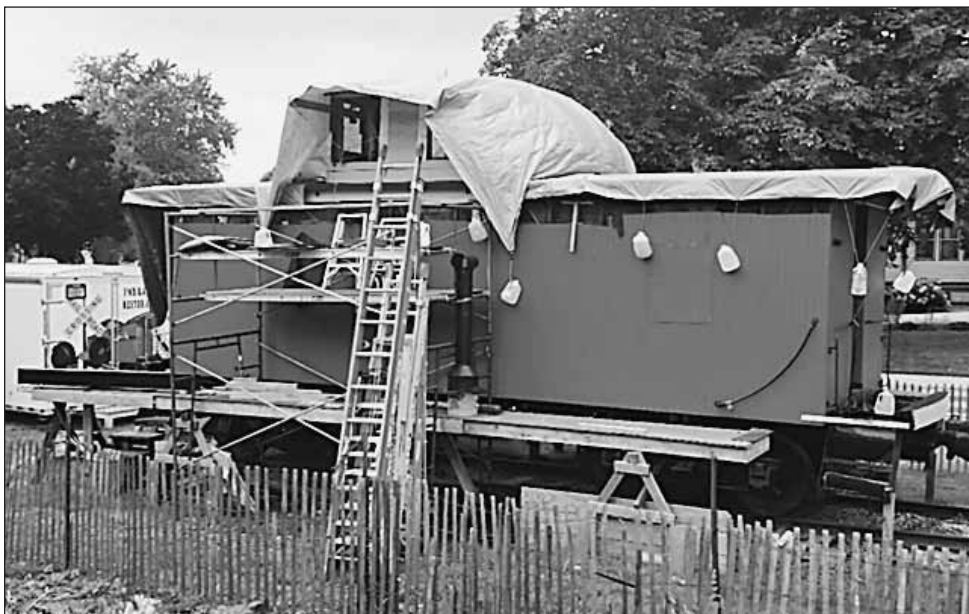
Organizers of the caboose renovation project are seeking additional donations to complete the project. The caboose project is making progress and in the next couple of weeks you will see significant changes.
