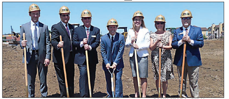
FIRST DIG: Tim Lyons, TTCU president and chief executive officer, along with TTCU executives and board members joined community dignitaries to break ground for the new facility June 25. From left are Shelby Beil, chief financial officer; Doug Aldrich, executive vice president/chief operations officer; Dan Bowling, chief information officer; Lyons; Laura Miller, chief human resources officer; Stephanie Jones, chief risk officer; and Charles Chastain, sr. vice president of lending.
