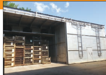
Dry Kiln & Hurst Gas Boiler 20,000 board ft. per side!
