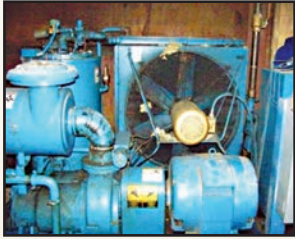
100HP Quincy Q490 Air Compressor
