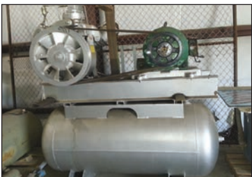
25 HP Ingersoll Rand w/30 HP Motor & 150 gal. tank (used)
