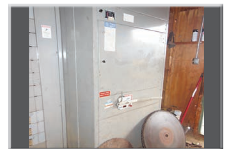
WESTINGHOUSE 1600A Main Switch
