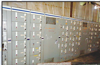
Large Amount of Motor Control Centers
