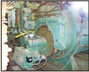
Two (2) Kewanee Boilers 650HP
