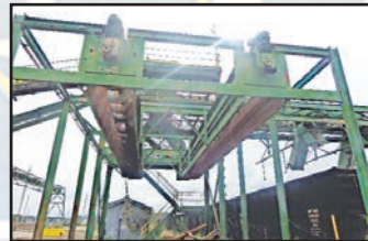
Overhead Truck Loading System
