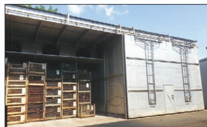
Dry Kiln & Hurst Gas Boiler 20,000 board ft. per side!
