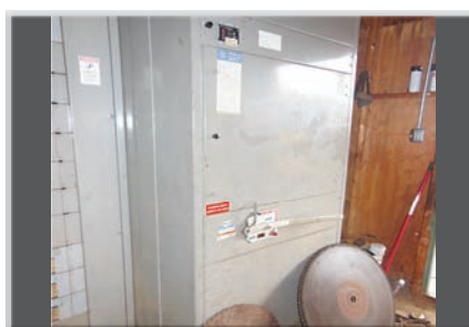
WESTINGHOUSE 1600A Main Switch
