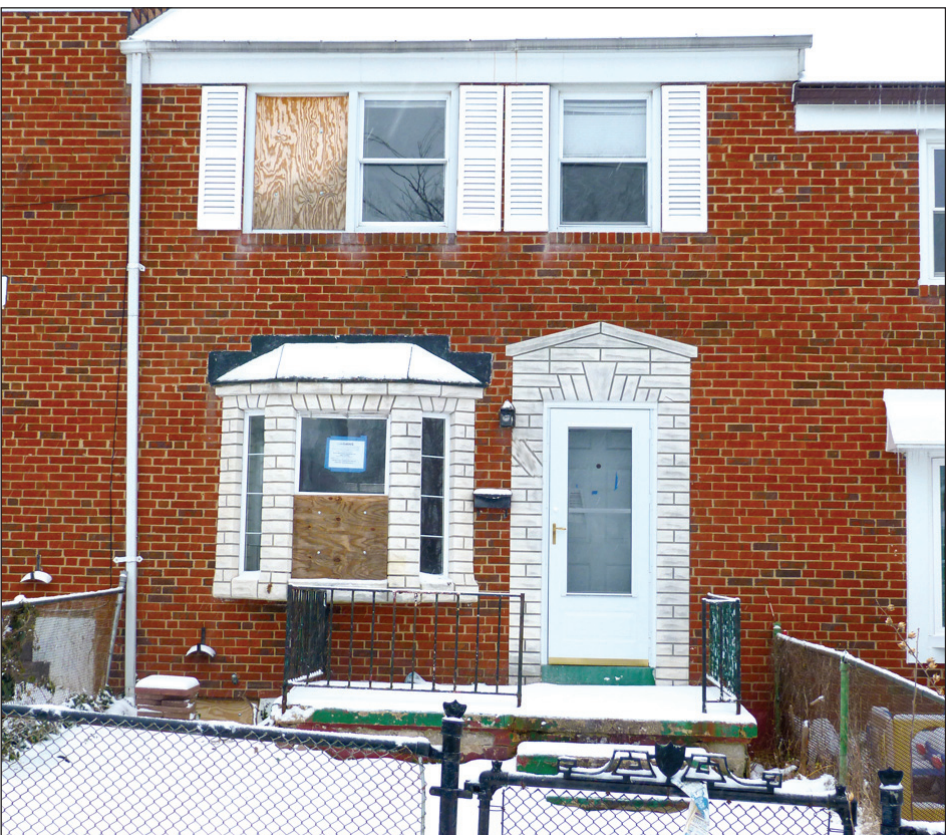
This vacant rowhouse in Middlesex is just an example of the many homes throughout southeastern Baltimore County which are left vacant for long periods and can attract squatters, drug users or rats when people begin dumping on the property illegally. File photo.
