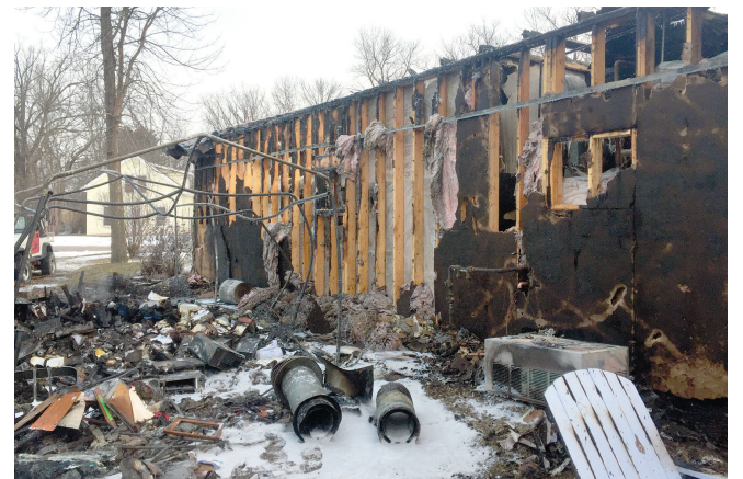
According to Deerwood Fire Chief Mike Bodle, the fire started between Salem WEST and the neighbor's garage in a temporary structure that was not owned by Salem WEST.
