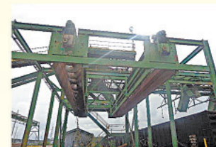
Overhead Truck Loading System
