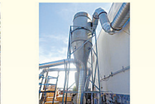
Dust Collection System
