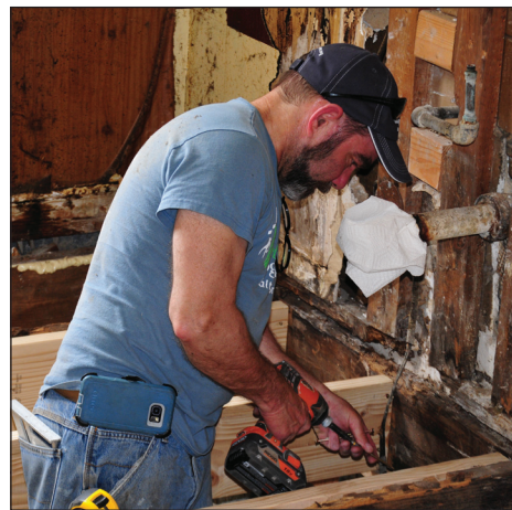
Rebuilding Together Baltimore volunteer Greg Oates replaces floor joists in a Turner Station home.
