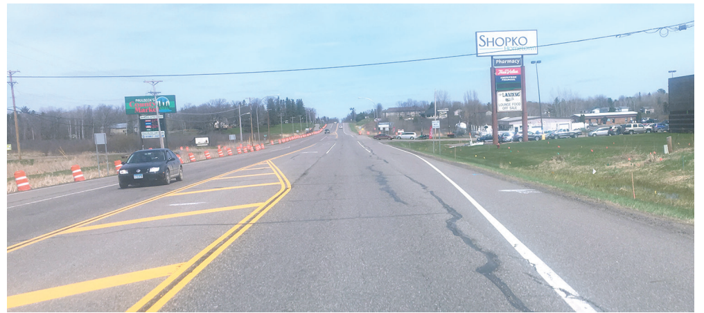
Construction for a new roundabout is located on Highway 169 near Red Oak Drive/Southgate Drive south of Aitkin at the entrances to Paulbeck's County Market and Shopko.
