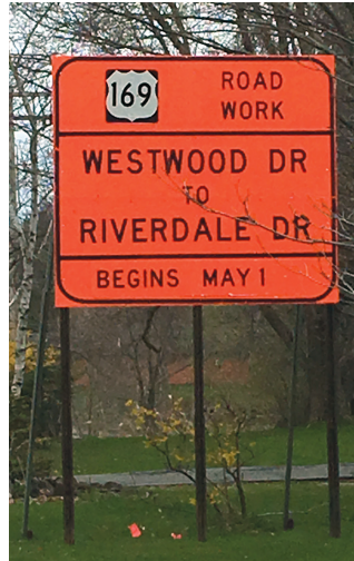
Construction for a new roundabout south of Aitkin began May 1. Schwartz Photo
