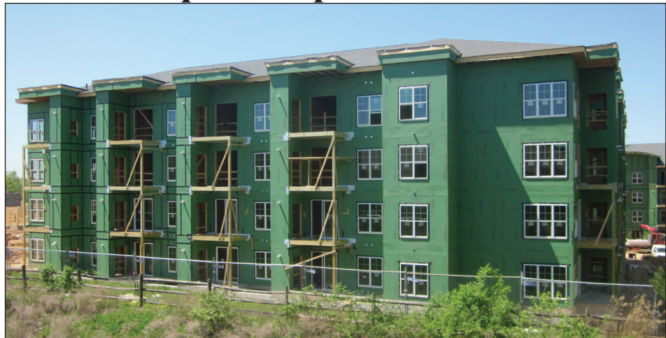
The Overlook apartments, which are visible from I-95, are currently under construction.
