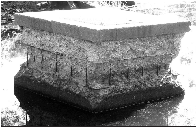
Crumbling gatehouse at Powell Pond in Tolland. Victim of pyrrhotite in concrete? Bill Hoboth photo
