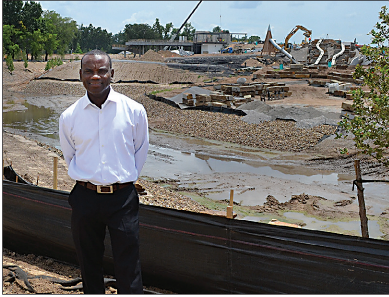
CONSTRUCTION OVERVIEW: A Gathering Place for Tulsa Director Tony Moore stands near the north end of the Gathering Place. Behind him are Peggy's Pond and the Boathouse. Moore came to Tulsa from Orlando and officially began his role in August of last year.
