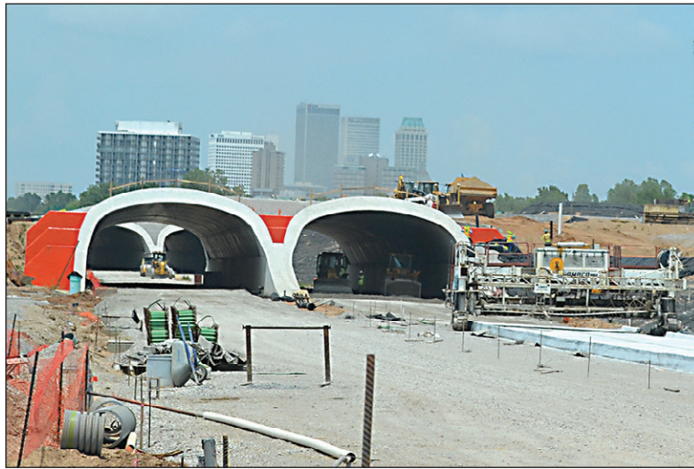
LAND BRIDGES: A view of the land bridges that will create tunnels on Riverside Drive. The bridges will extend the park over the street and connect it to the Arkansas River. The tunnels will feature LED lights and have a European design element. Care is also being taken to engineer the bridges to minimize traffic noise from Riverside and to use vegetation and the landscape to muffle sounds.
