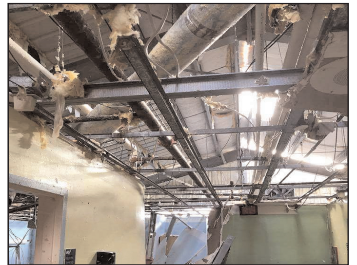
COURTESY PHOTO: LA'MOR FRET THIS PHOTO OF THE SEAVIEW HOME FOR THE AGED AND INFIRMED IN ST. THOMAS IS JUST ONE EXAMPLE OF THE LEVEL OF DESTRUCTION AND DEVASTATION BY HURRICANE IRMA.
