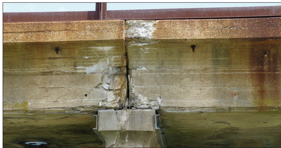
Residents living around the bridge have grown increasingly concerned about things like crumbling and spalling concrete at several places along the span.
